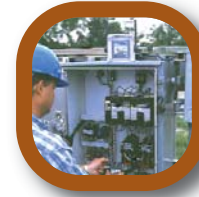
4501 Pump Station Flow Monitor
