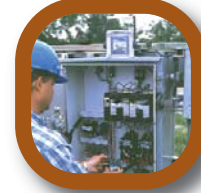
4501 Pump Station Flow Monitor
